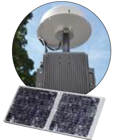
Mast mounted Outdoor Unit with solar panel
